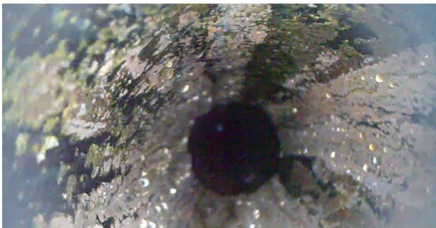
Scale build-up within wellbore
